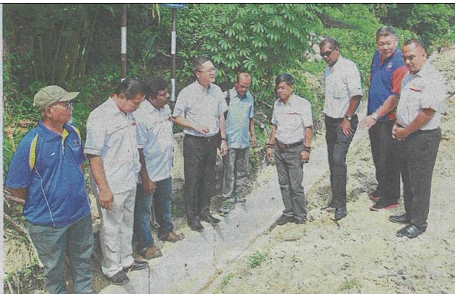
Lai (fourth from left) at the Taman Saga drainage project site in Ampang Jaya, Selangor. With him is Abdul Razak (second from left).
